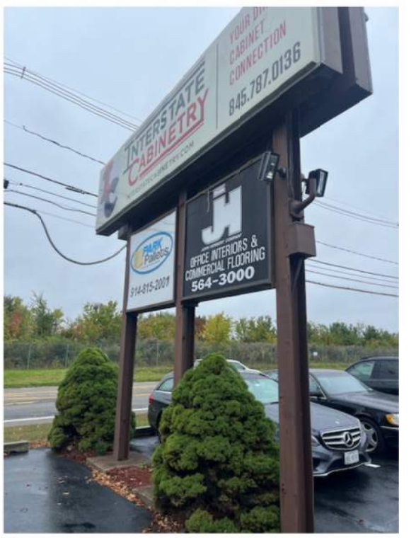
EXISTING EXTERIOR LIGHTS ON EXISTING SIGN
